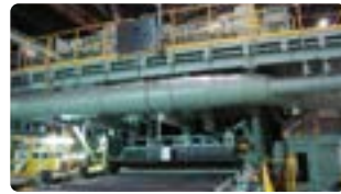
Plate mill: Cold leveller
